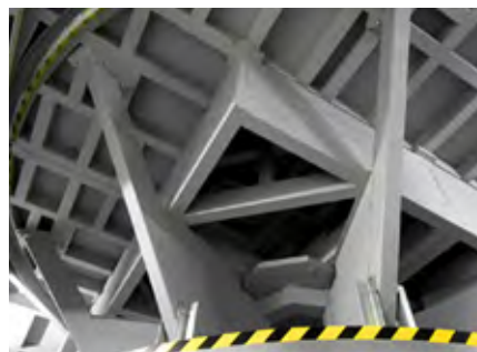
View of the lower structure from the pit. This entire structure rotates in the new system.
