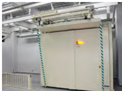
The door has been fully moved, waiting to be slid to the left (the lifter elevates)
