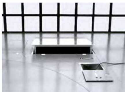
The hatch halted at the predetermined position. Another switch must be activated to close it entirely.
