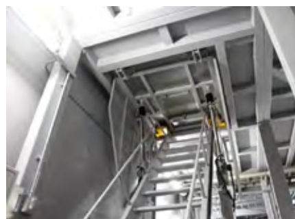
View of the stairway seen from the pit side, a safety-first electric open/close structure.
