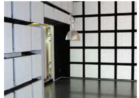
The lighting can be lowered to this level for easy maintenance works.
